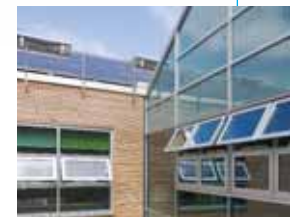
Automatic opening vents in facade
