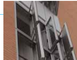
Glazed smoke and heat exhaust ventilation (AOV)
