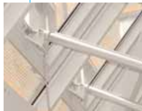
Automatic opening vents in rooflight
