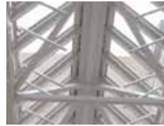
Smoke and heat exhaust ventilation
